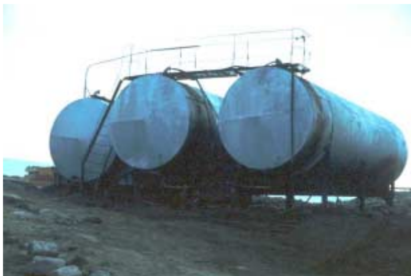
Photo 8: Fuel storage at Novolazarevskaya
